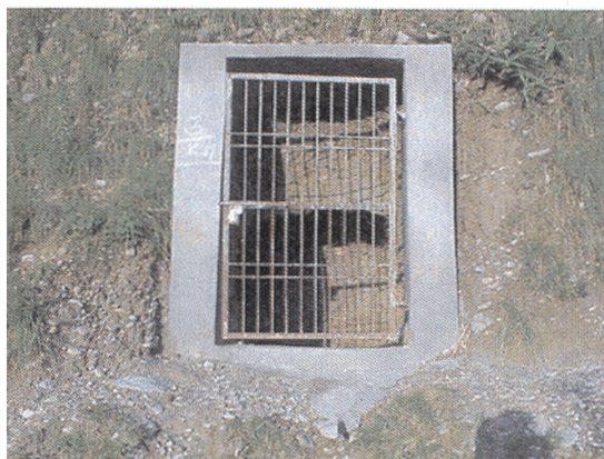
Fig.7 Iron door and lock guard water in khatri
